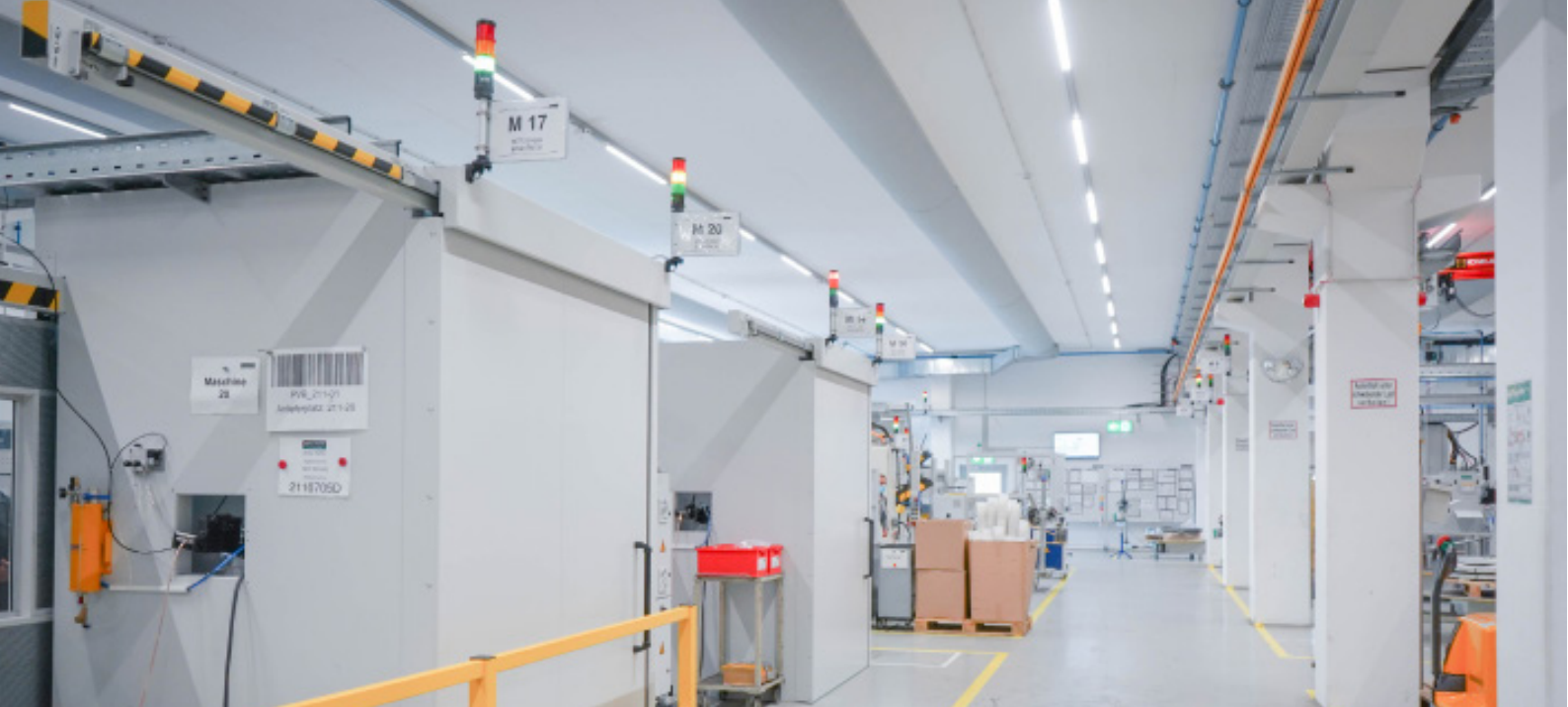
At the moment, 60 machines at Eberle Rieden are equipped with SmartMONITOR. This equates to more than 95% of the entire plant.
